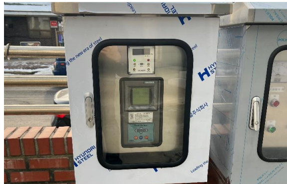
Backwash integrated flowmeter and pH display panel installation
